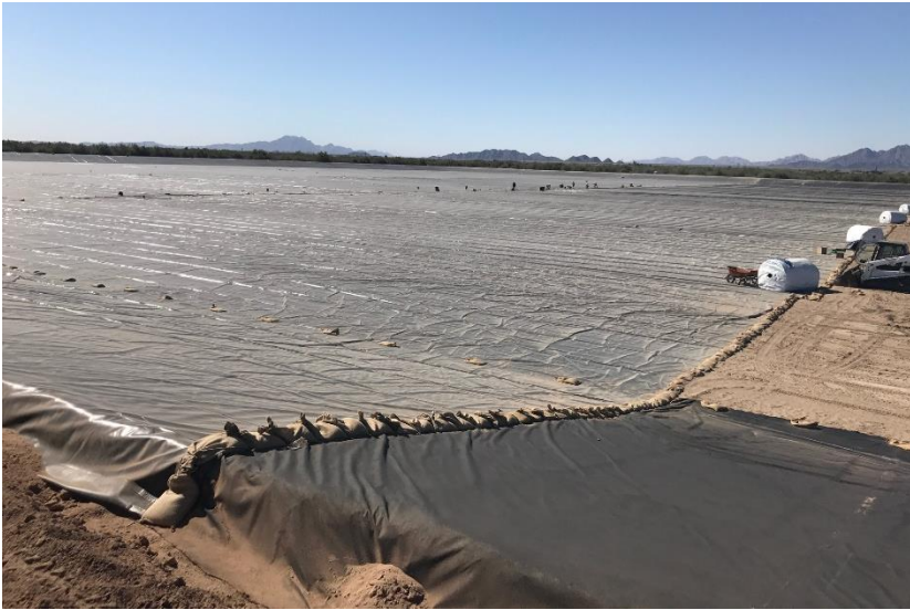
Positioning ballast immediately following each RPP panel deployment due to high wind conditions.
