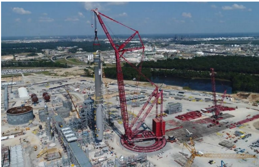
Figure 1. Third largest ringer crane in the world operating on a multi-axial geogrid stabilized working platform in the US
