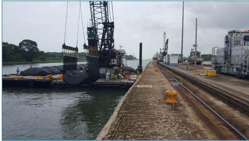
Figure 2. 90 Ton Geobag Prepared to be Placed in -20.0m of Water at Gatun Locks
