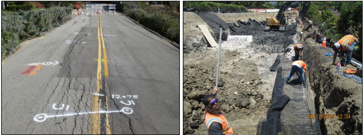
Photo 1. (Left) Arcuate cracking and failure of roadway surface prior to temporary realignment.
