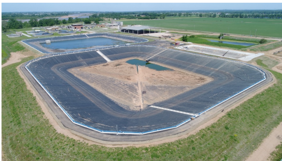
Figure 2. Haikey Creek WWTP Geomembrane Lined Flow Equalization Basins
