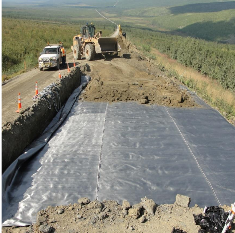
Figure 1. Installation of Wicking Geotextile to Mitigate Frost Boils at Beaver Slide of Dalton Highway, Alaska
